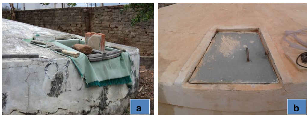
Figura 33 - (a) Cisterna rachada com tampa inadequada, (b) Cisterna com tampa adequada
